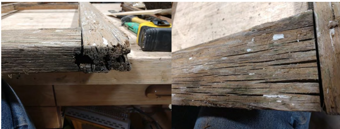
Photos of historic wood window sash that experienced years of neglect, lack of maintenance, and weathering of material.
